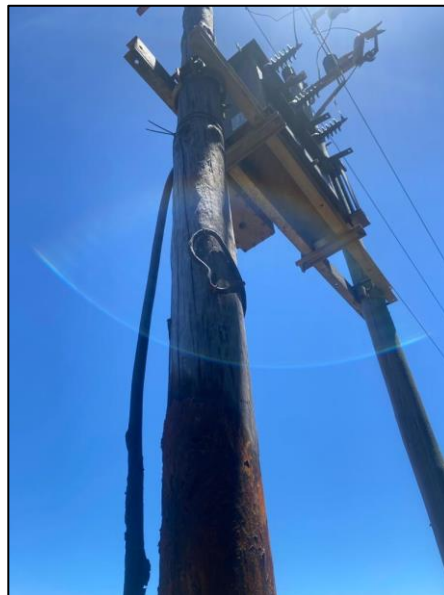
Figure 13. H Poles are regularly greased.
